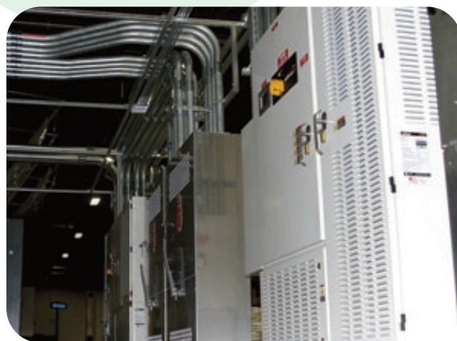
Inverters help turn the solar energy from the roof into usable electricity in the building.
